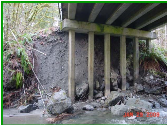
A view under the bridge before the repair project reveals severe erosion caused by flooding in 2009.
