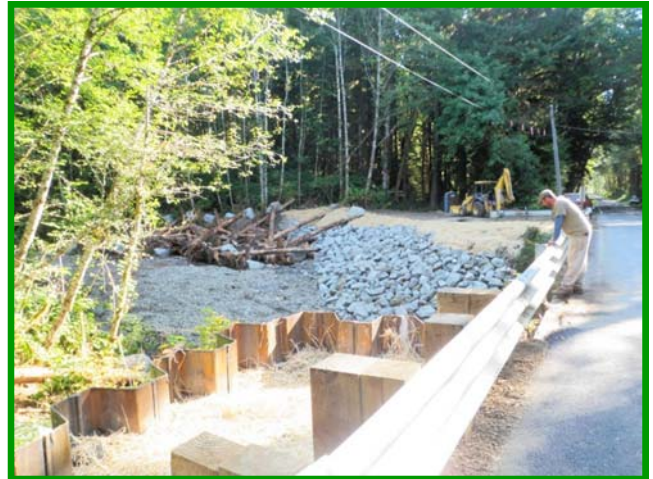
This view of Willoughby Creek Bridge shows many elements of the project — new sheet pile wall (foreground), and stream bank armoring and engineered logjams (background).
